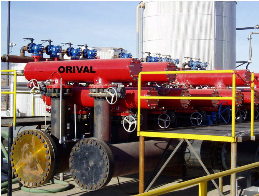
Figure 1. Orival filtration system.
