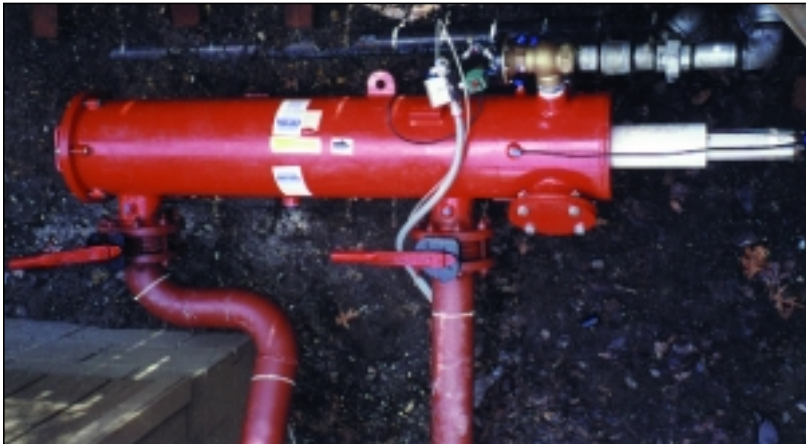
Model OR-04-PE filtering 350 gpm of canal water prior to distribution to sprinkler heads. A similar installation was made of an OR-08-PS filter for 1300 gpm of pond water.
