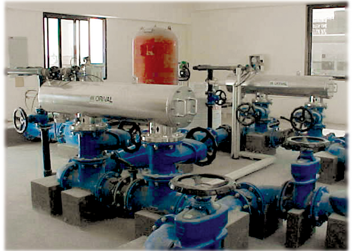
Two ORI-08-PS-S stainless steel units filter diluted sea water to protect golf course sprinkler systems
