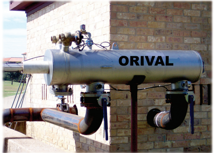
One ORI-06-PE-S stainless steel filter keeps Four Seasons' golf course irrigation system clog-free
