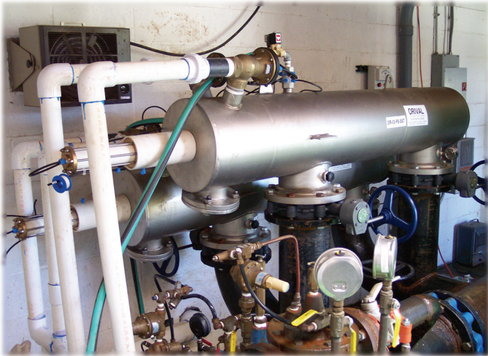
Two ORI-08-PS-S stainless steel filters keep Four Seasons' golf course irrigation system clog-free
