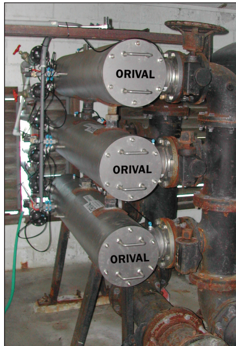
A bank of 3 stainless steel model ORI-06-PE-S filters rated at 2000 gpm protecting Bodega's sprinklers
