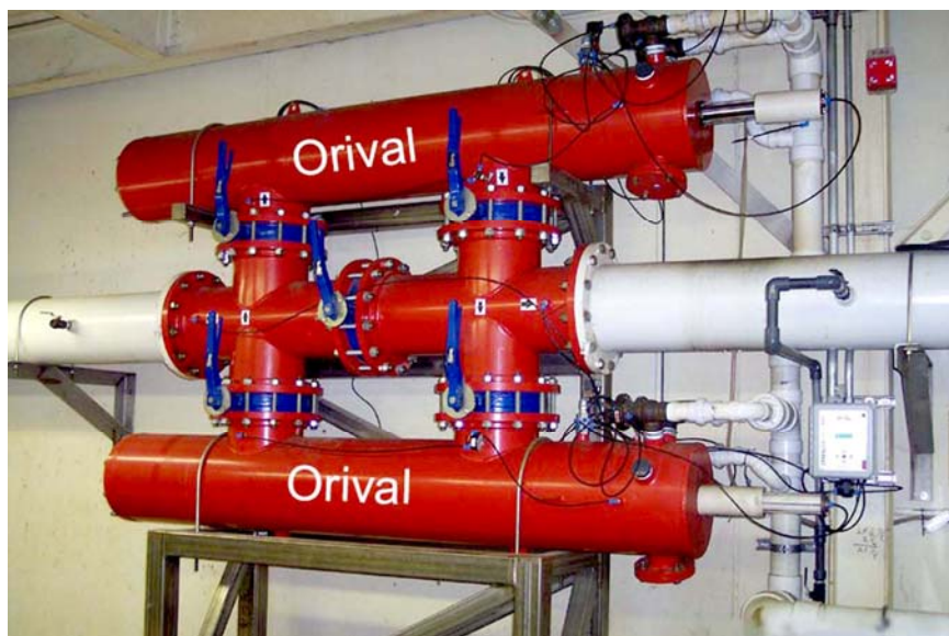
Figure 1. Filtration system: Two Orival OR-12-PS filters with manifold.
